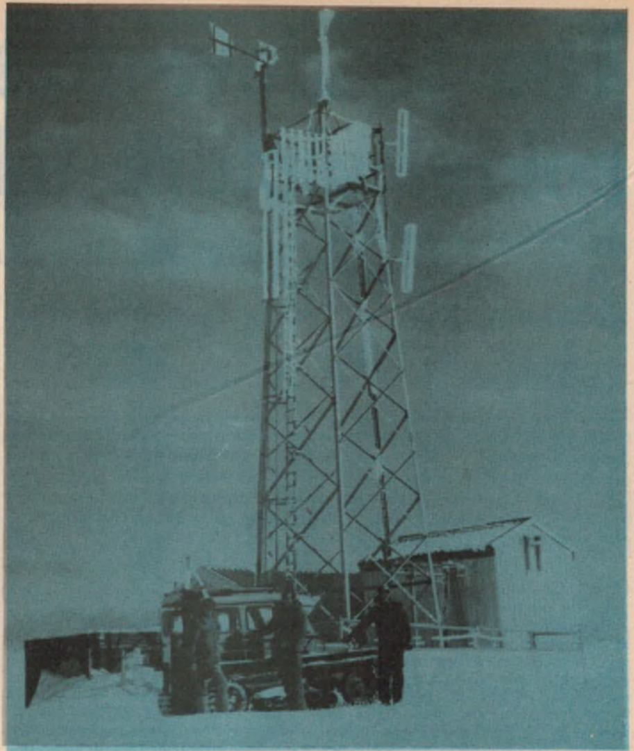
Field staff go by Snow-cat to the Mt. Hotham exchange. Note the build up of ice on the upper sections of the mast's structure.
