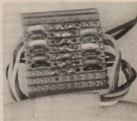
ABOVE: This photograph shows how we terminated the transmitter loop onto a small piece of Veroboard.
