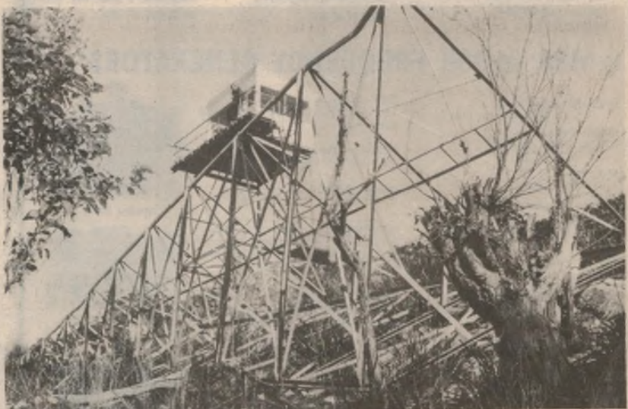
The vandalised tower lying where it fell, with some of the distorted members clearly visible. The tower probably can be repaired, but the wind charger was a write-off. The building in the background houses the repeater.
