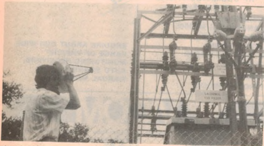
This posed picture illustrates how the ultrasonic detector might be used to check a typical sub-station installation. Note that the operator can work from outside the boundary fence, which may often be quicker and more convenient than having to obtain permission to enter the area.
