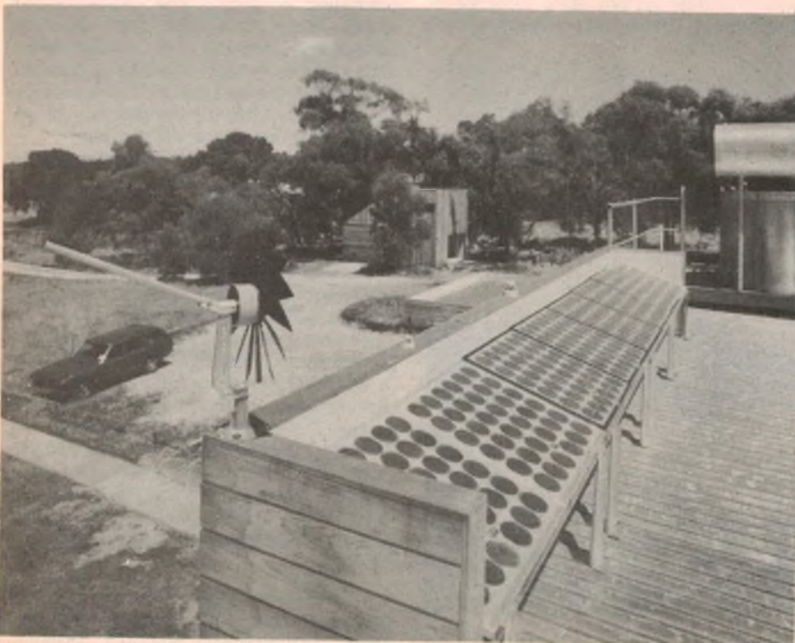
Eight solar cell arrays each provide 2.5A at 14.5V, with a total capacity of 20A.
