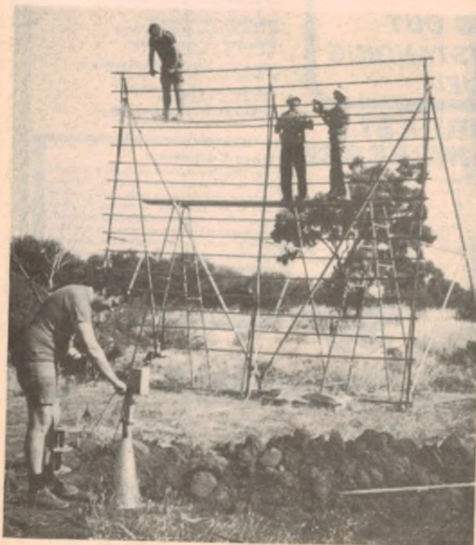
The curved reflector screen for the Hills satellite TV system is shown here under construction.
