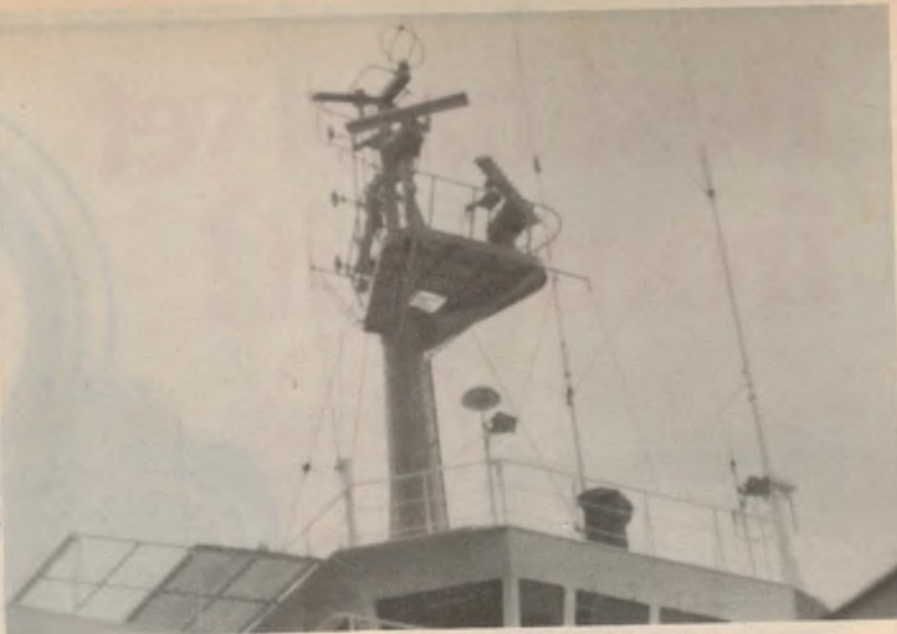
Cluster of antennas on the MV Zim Kaohsiung is typical of modern vessels.
