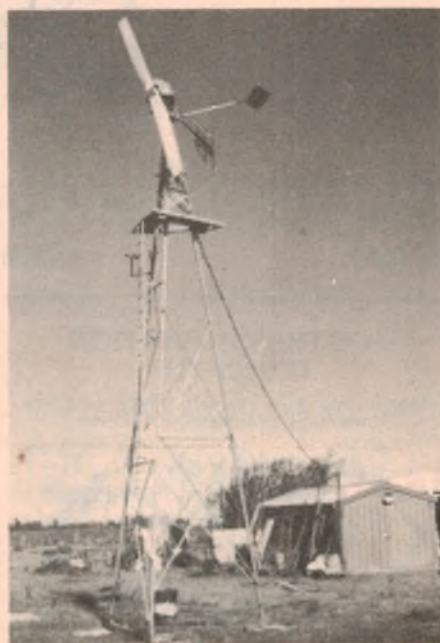
In a 40km/h wind the author's installation delivers 13.8V at 18A (250W).
