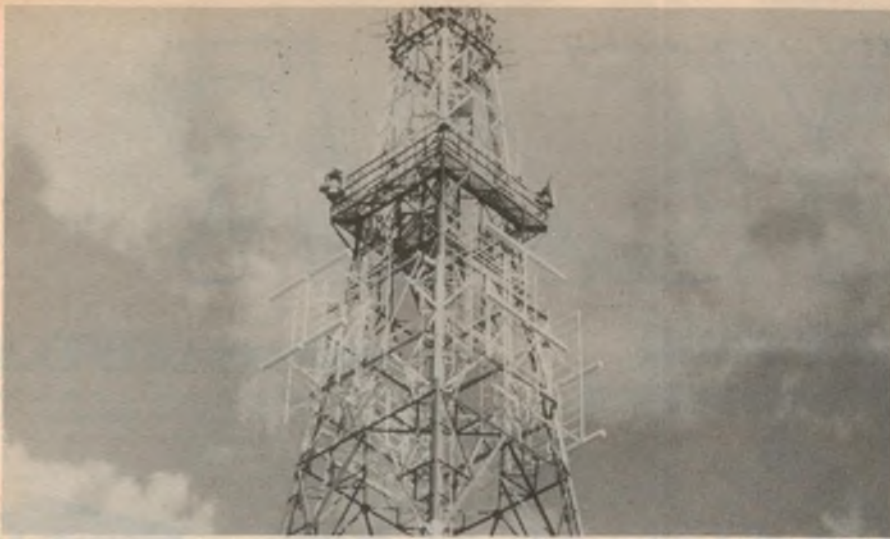
Most TV antennas are variations on the basic dipole antenna as described in this article. This large array is for Channel 0 in Sydney. The large dipoles can be easily recognised, ie, the hefty lengths of horizontal pipe painted white.
