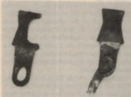
This view clearly shows the damage to the switch contacts.
