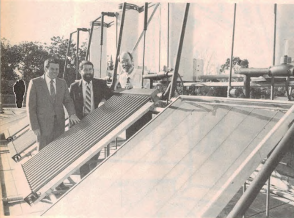
Conventional and glass tube collectors on the roof of the Physics Building.
