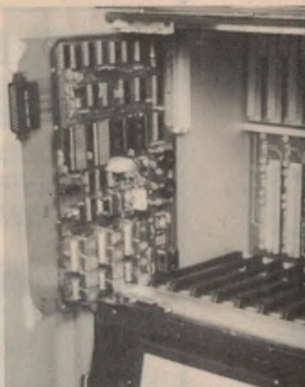
Interior view of an on-site controller, adjacent to a set of traffic lights.
