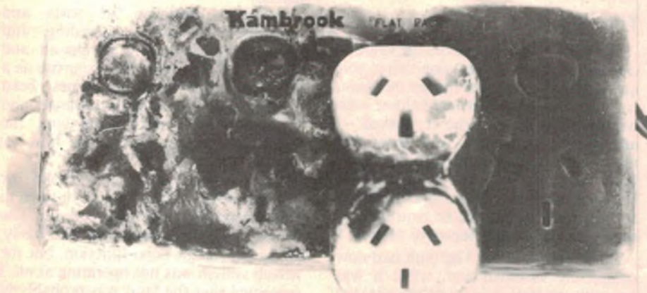
Pongo's legacy — the blackened power distribution panel.
