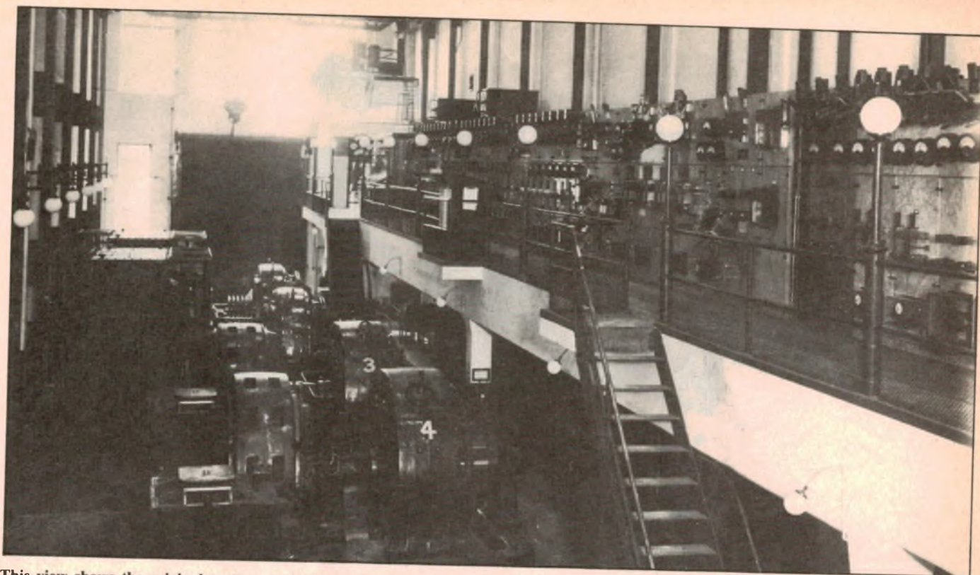
This view shows the original motor-generator sets in the Clarence Street sub-station, before their replacement by the mercury arc rectifiers and transformers.
