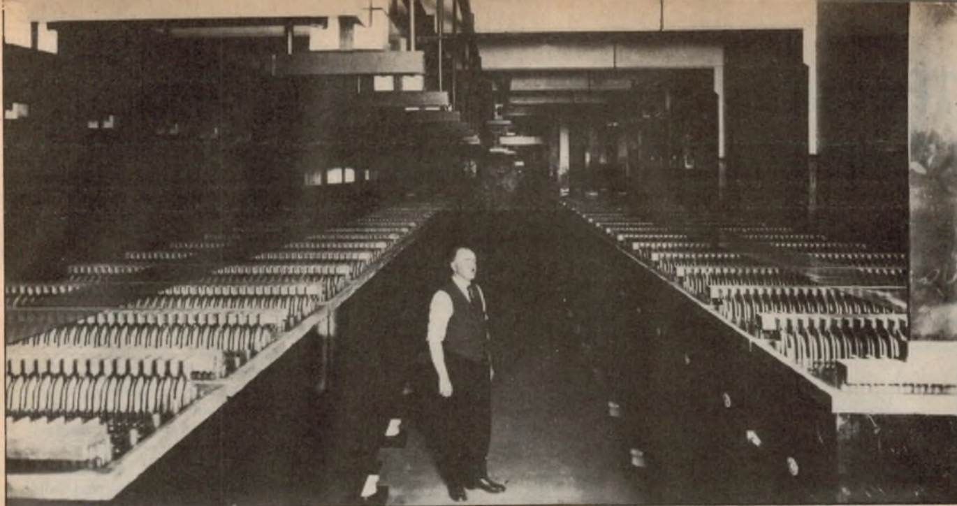
These battery banks were used to buffer load variations and occupied an entire floor of the sub-station.
