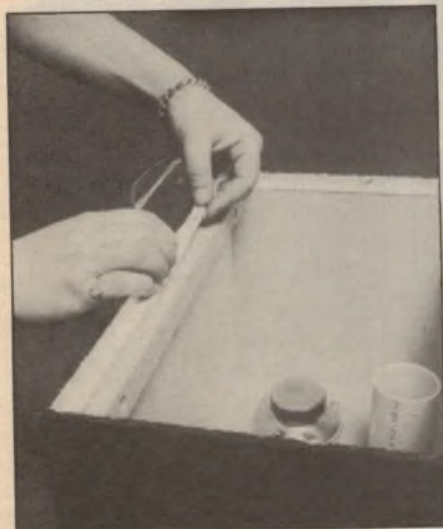
Draft exclusion tape is applied to the cleats to provide an airtight gasket for the rear panel.
