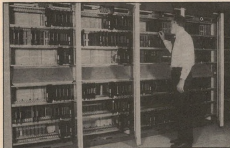
An STC System 12 ISDN facility installed at the Research Laboratories of Telecom Australia, in Clayton Victoria. Courtesy STC)
