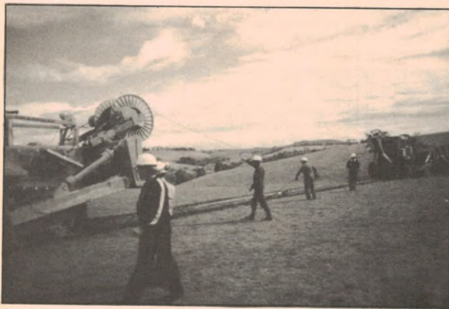
A Telecom Australia team laying fibre optic cable into the ground, using a direct ploughing technique. (Courtesy Olex Fibre Optics)
