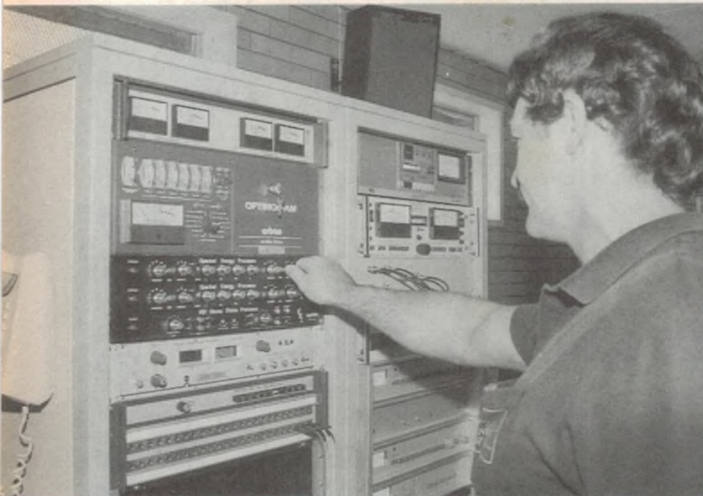
Close-up of the audio control racks in the transmitter room, with chief engineer Allan Bone making an adjustment.
