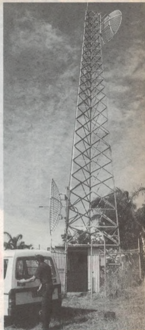
2MW's microwave relay station at Terranora. The top dish points to the transmitter site.
