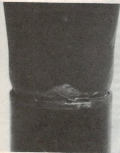
Fig.1A: A common problem with metallising. Not only has the base become loose, but the earthing wire has lost reliable contact with the shielding.
