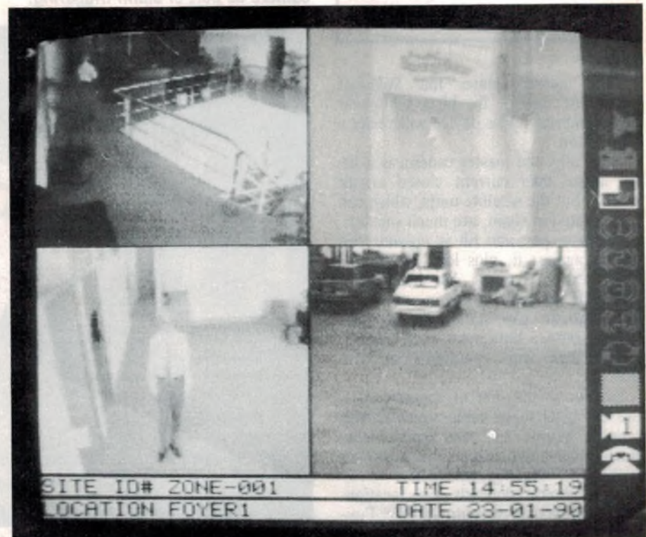
Typical company installation, as covered by four cameras at maximum resolution. Note icons at right of screen, each depicting functions available.
