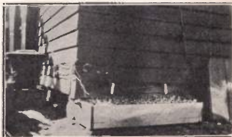
Typical Chemical Rectifier outside the shack (Note the pole transformer)
