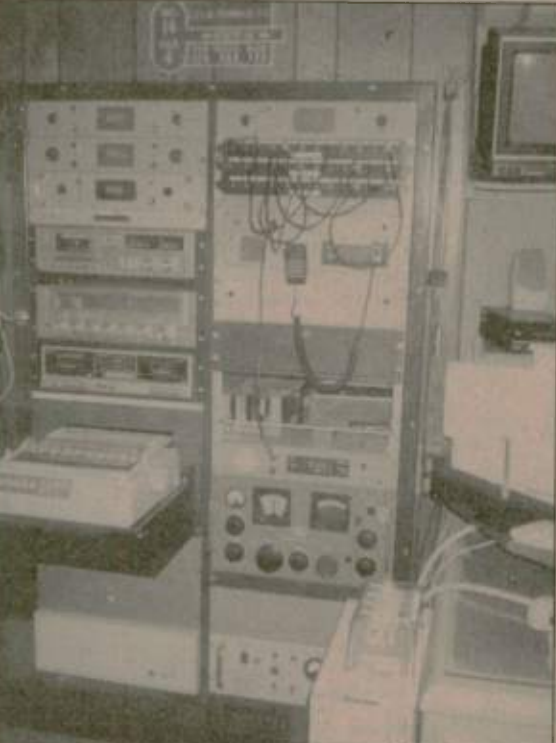
This equipment rack is built into a false wall, which helps to keep the wire clutter hidden.
