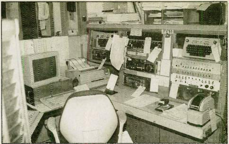
One of the CW consoles at KPH — all the equipment is still in place, and there are undelivered messages in the rack on the left.
