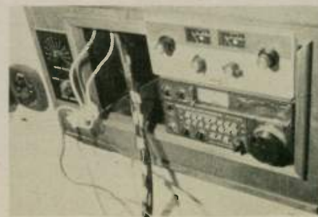
The best time to run the wide ground system is when initially installing your equipment — here, ICOM 720 and Cubic tuner.
