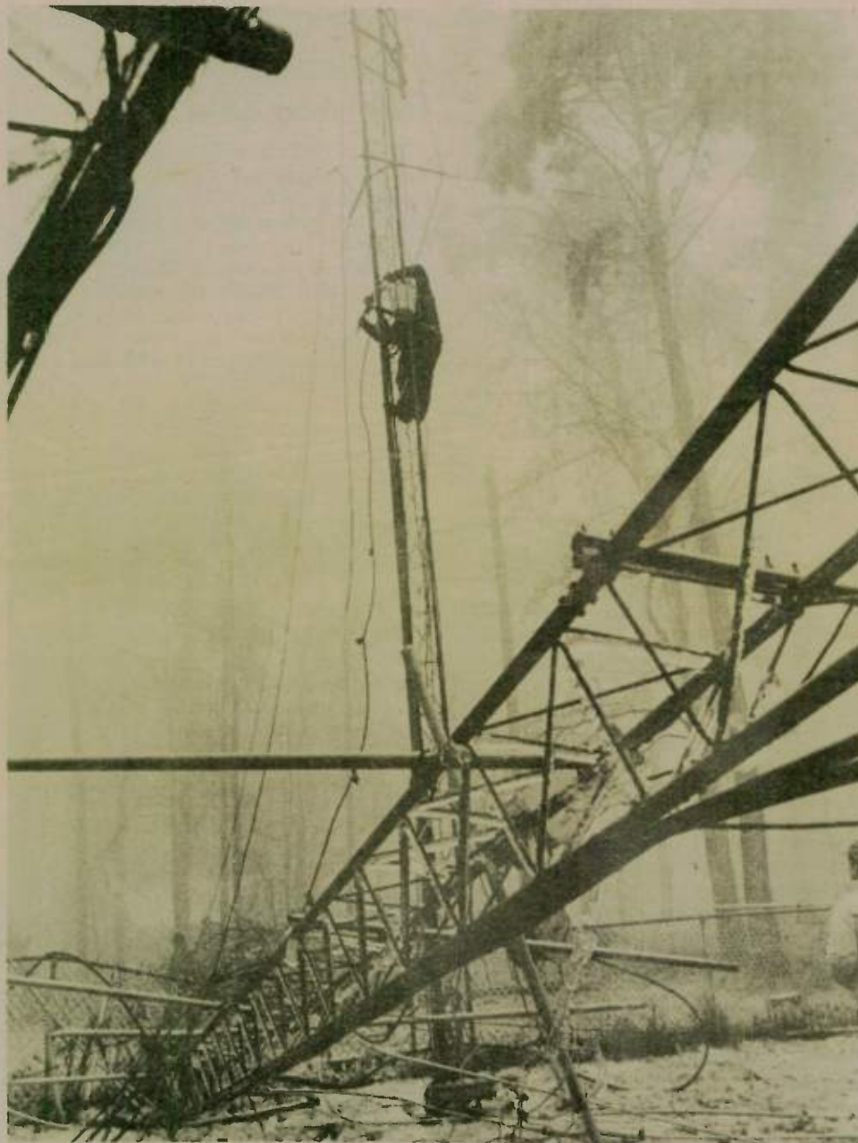
Clyde Rutherford, WA4JUM works on emergency repairs to central Alabama's 34-94 repeater tower, which went out of action when a tree limb fell across a guy wire and took the upper two-thirds of the tower down. (Photo by Joe Veras, N4QB)
