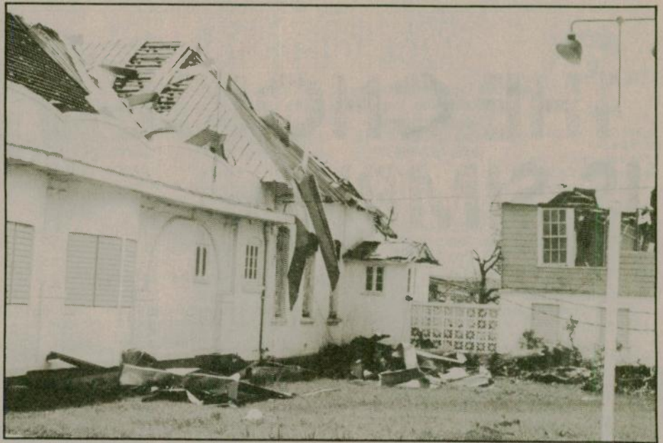
The Salvation Army HQ in Kingston, Jamaica suffered much damage.
