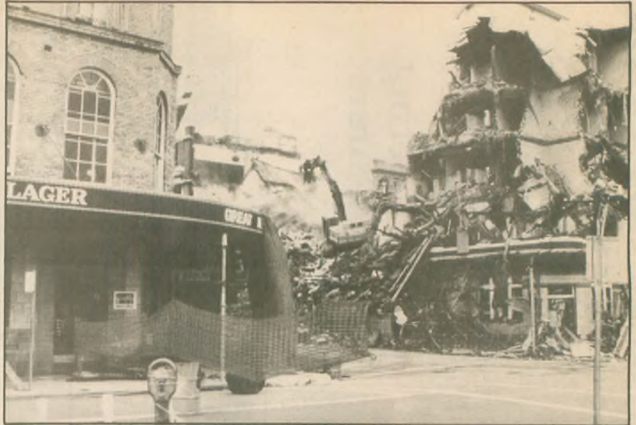
The partially collapsed George Hotel
