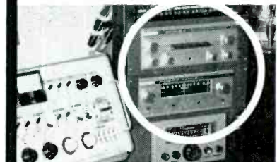
Perfect partners! Rack-mounted solid-state Altec 360A PLAYBACK Amplifier works with Altec 314A FM Multiplex Tuner at Sim-O-Rama Sound Recording Studio.
