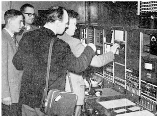
Roy Coyston, a blind member of the Walthamstow and District Tape Recording Society being directed round the Coppermill telephone exchange by M. Dudley. Members C. Stares and T. Norton look on.
