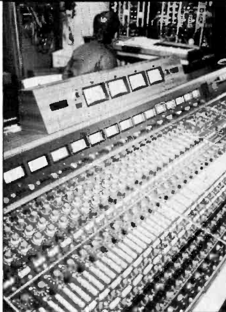
Control room of Studio One Audiofilm SA
