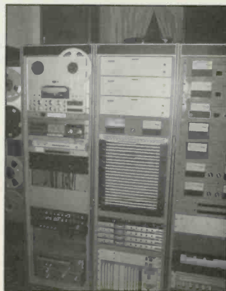
Distribution and monitoring racks.
