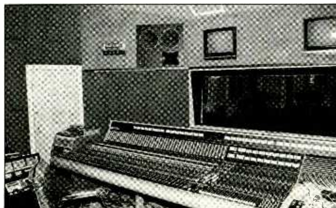
Control room A1 with modified TSM console
