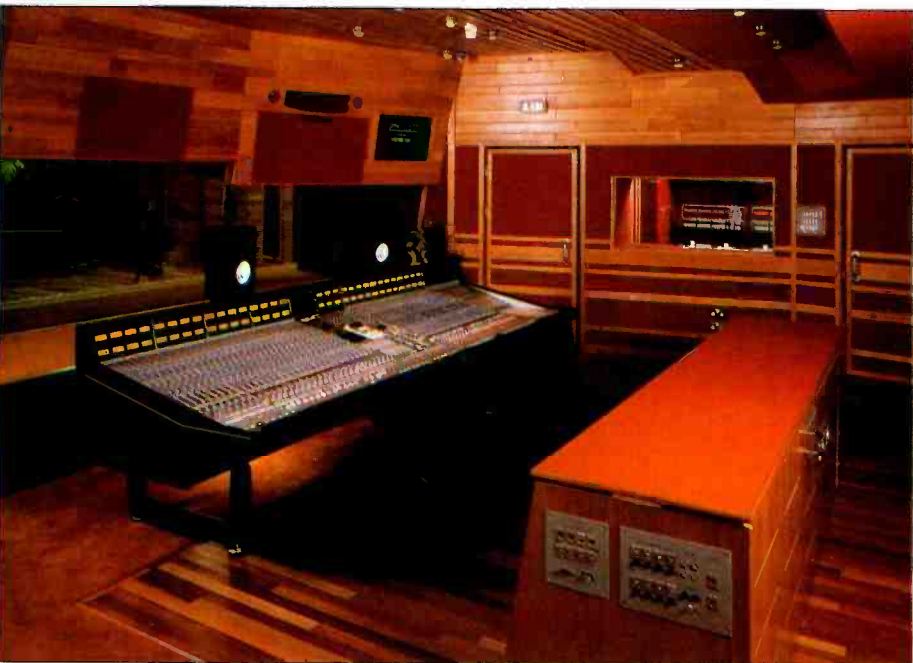
Control Room One
