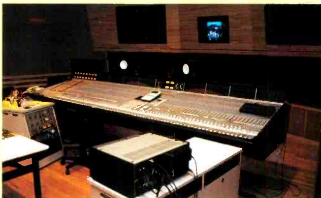
▲ Tokyufun Recording Studios, a new state of the art three-room facility in Tokyo, has recently opened with G Series consoles. Each control room is identically equipped with SL 4064 G Series consoles and Sony PCM 3348 tape machines to provide uniform sound control.
