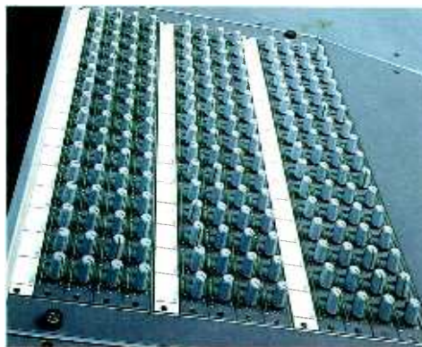
▲ The Real World Automated Send Matrix installed in the 80 channel G Series console at Real World Studios, Box, England
