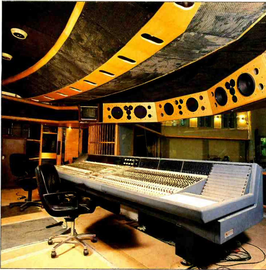
Interior of the Main Hall Control Room
