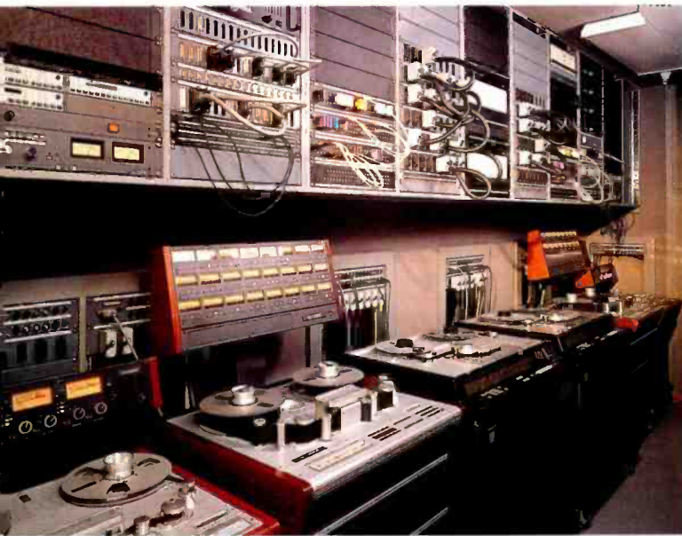
Sony 3348s, Studer 827 and 820 machines in the common equipment room. Note the comprehensive patching arrangements above the machine bay
