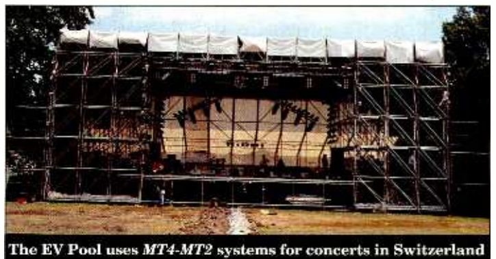
The EV Pool uses MT4-MT2 systems for concerts in Switzerland
