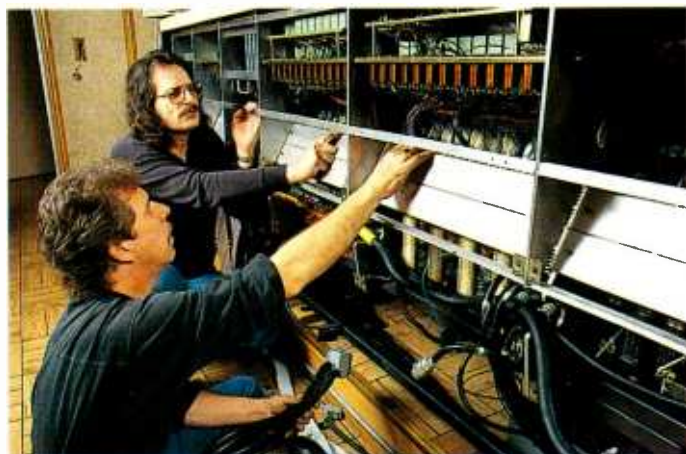
Fred Hill (left) with Sunset Sound's Chief Engineer, Mick Higgins, checking out rear-panel wiring and logic interconnections for the enhanced solo-AFL systems fitted to the revitalised Neve 8088 console
