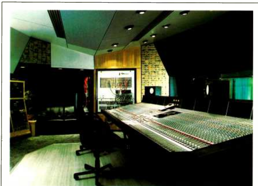
Control room studio 1 with SL9072-J console
