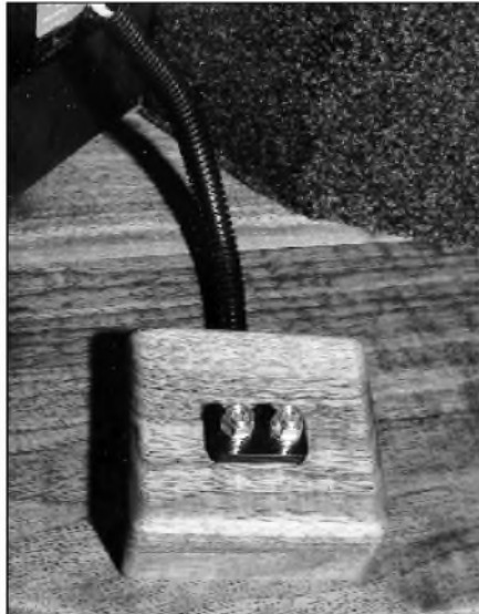
PHOTO 33: Terminal block mounted.
