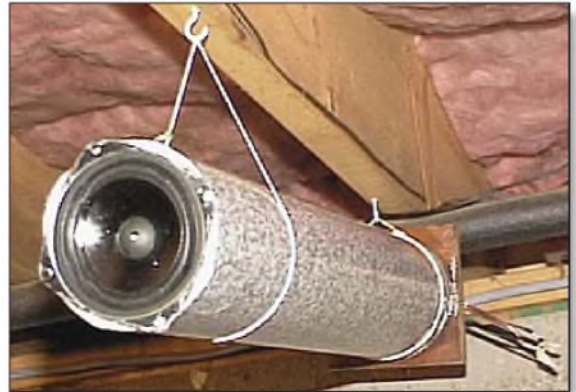
PHOTO 1: The completed speaker in place.
