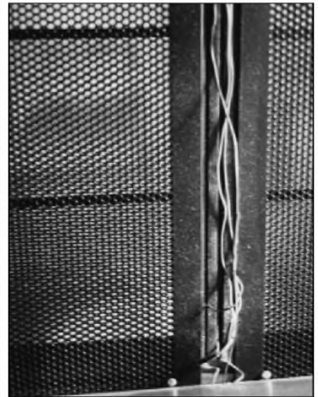
PHOTO 5: Wiring of the adjacent panels.
