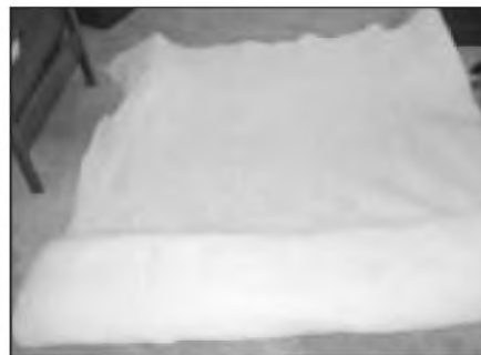
PHOTO 14: Quilting material spread out and being rolled into a width for V1 cavity in the T-line.
