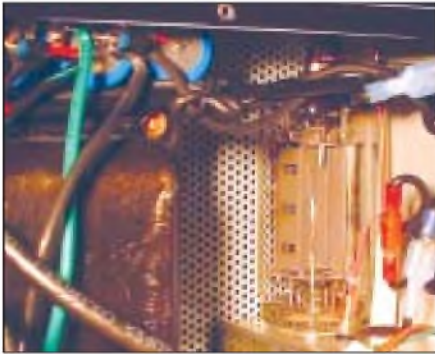
PHOTO 7: The 6KG6A is mounted in the front of the enclosure.
