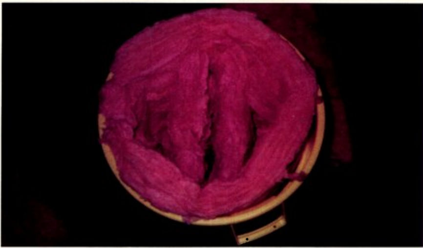
THINK PINK: Installing the two vertical fiberglass sheets. Note the spaces between pieces.
