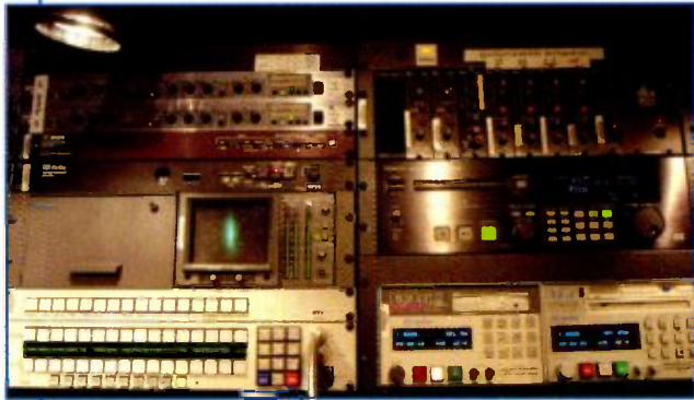
Due to space constraints in the mix room, rack gear is mounted in a bridge floating above the console.
