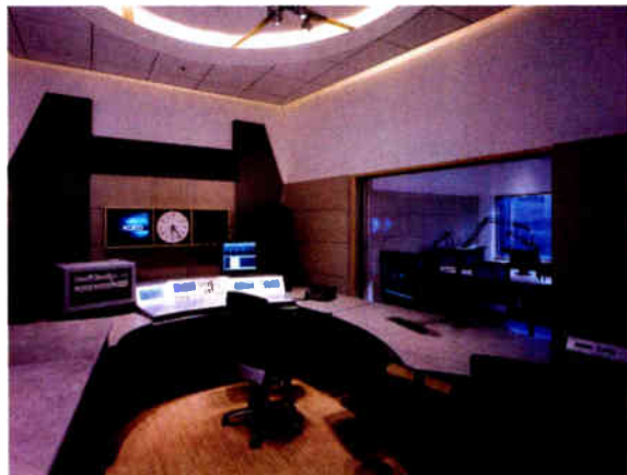
KQED's Master Control center features an ergonomic, spacious design built around a Studer OnAir 2000M2 console.
