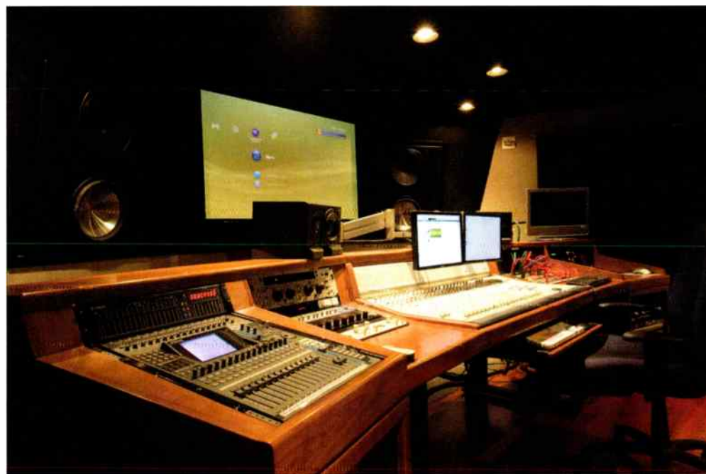
The main control room at SCEA’s Foster City, Calif., studio, with Digidesign Command-D console and Chris Pelonis-designed speakers
