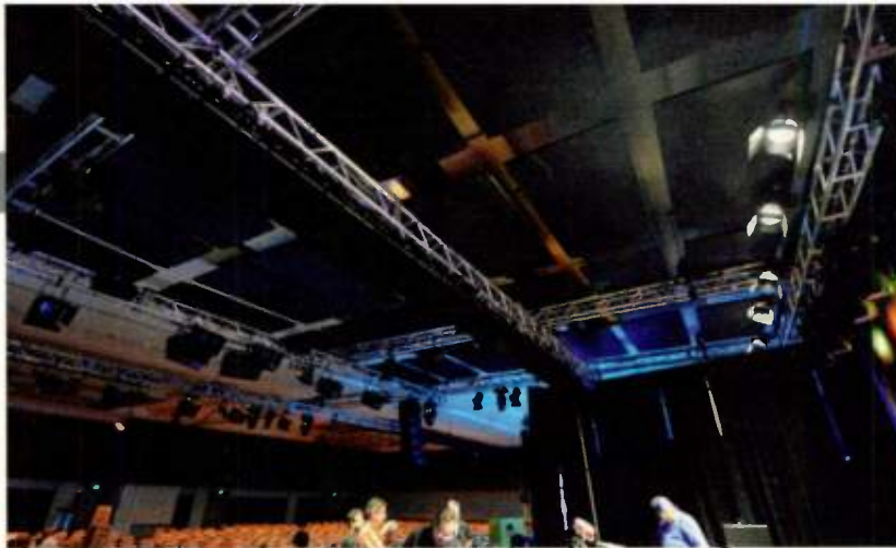
The ceiling of the Pacific Ballroom in the Anaheim Hilton was covered by a temporary installation of 200 custom GeerFab Acoustics MultiZorber panels.
