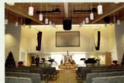
Legacy United Methodist Church recently had Bose Professional Systems RoomMatch components installed.
