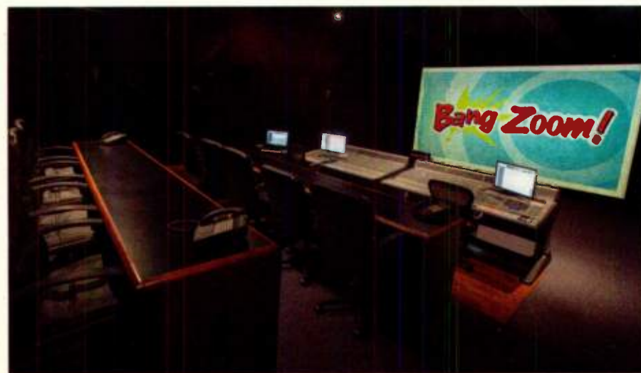
Bang Zoom’s Stage 3 is the facility’s largest room, sporting 7.1 surround monitoring.
