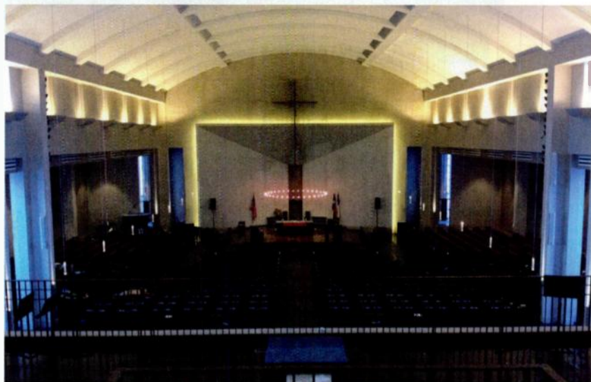
Digitally beam-steerable loudspeaker arrays, such as Meyer Sound's CAL system, installed at Trinity Lutheran Church in Spring, TX, can provide greater speech intelligibility than alternative speaker solutions in acoustically challenging house of worship environments.
